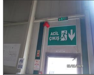
Photo of fire safety equipment Exit sign and luminescent light.JPG
