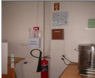
Photo of fire safety equipment NC7.14-CORRECTED-Alarm button was installed in the canteen area..JPG
