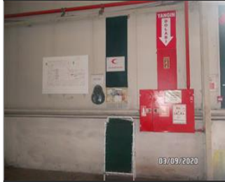
Photo of fire safety equipment Fire hose - first aid corner.JPG
