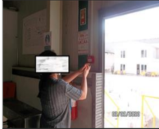
Photo of fire safety equipment Fire alarm tested.JPG
