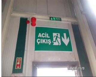
Photo of fire safety equipment NC7.14-CORRECTED-Visual and audible alarm exists on the exit doors..JPG
