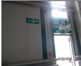
Photo of fire safety equipment NC7.14-CORRECTED-Both visual and audible fire alarm system was renewed in recent period..JPG
