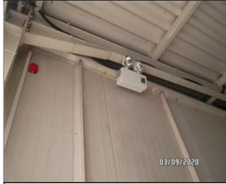
Photo of fire safety equipment Emergency exit light.JPG
