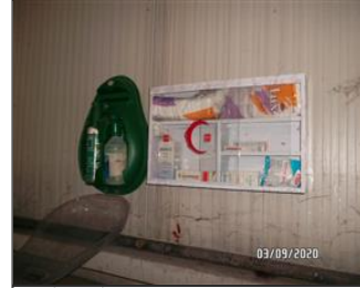
Photo first aid facilities First aid box- eyewash station.JPG
