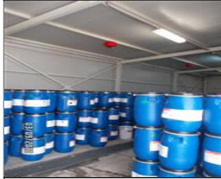
Photo of chemical storage room (if applicable) Chemicals storeroom.JPG
