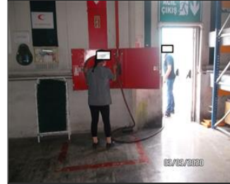
Photo of fire safety equipment Fire hose tested..JPG
