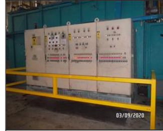
Photo of fire safety equipment Electrical protection.JPG
