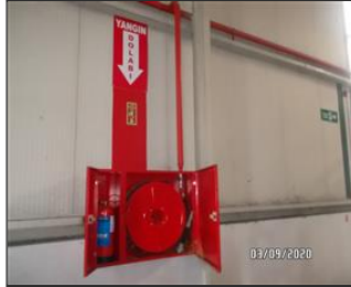
Photo of fire safety equipment Fire hose.JPG
