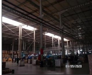
Photo of non-conformity NC7.25and7.1-PARTIALLY CORRECTED-Lighting was insufficient especially in the warehousing and roller .JPG
