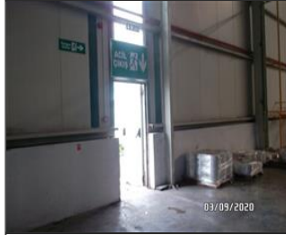
Photo of fire safety equipment Exit door.JPG
